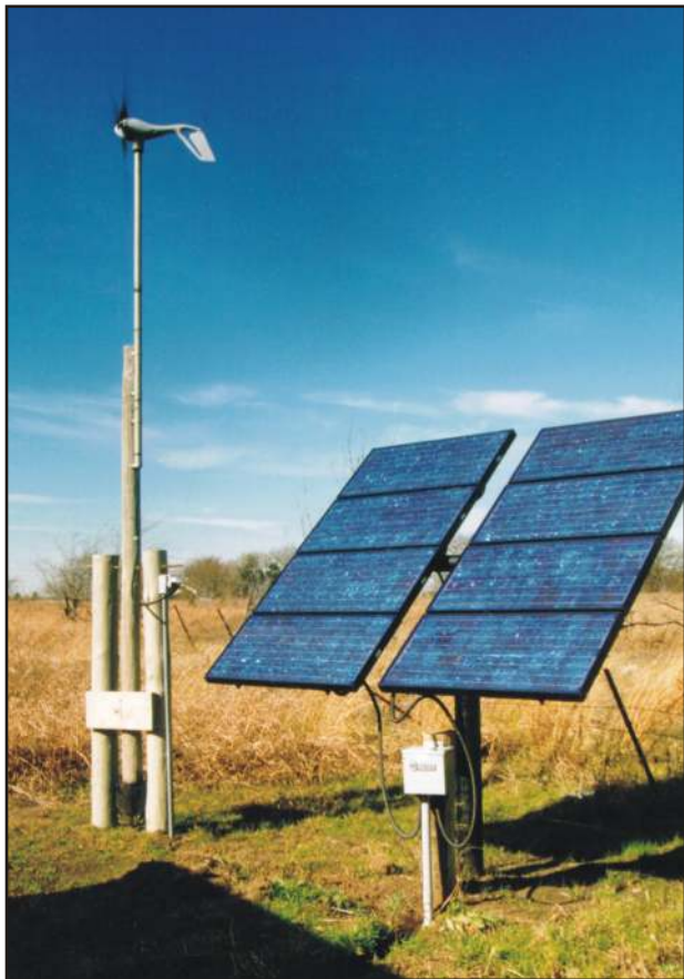
An Air 403 pairs with a PV system to supply a consistent supply of power for battery charging.
